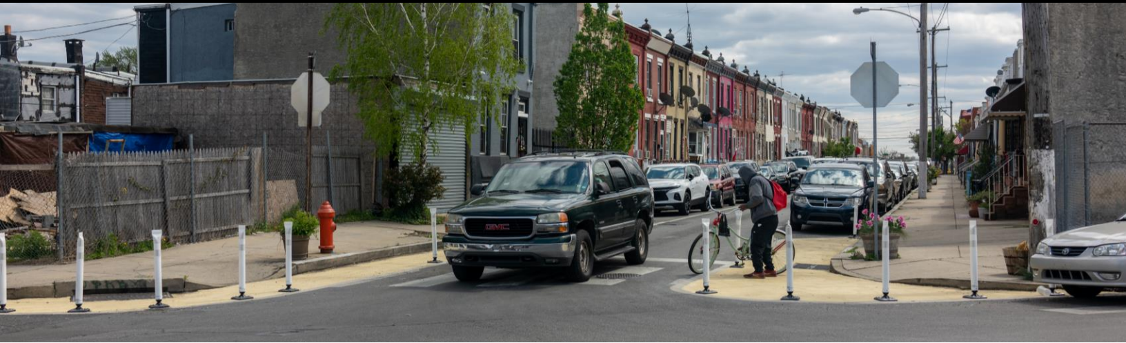
Painted curb extensions after construction, Glenwood Avenue, Tioga, and 3rd Streets, April 2022
