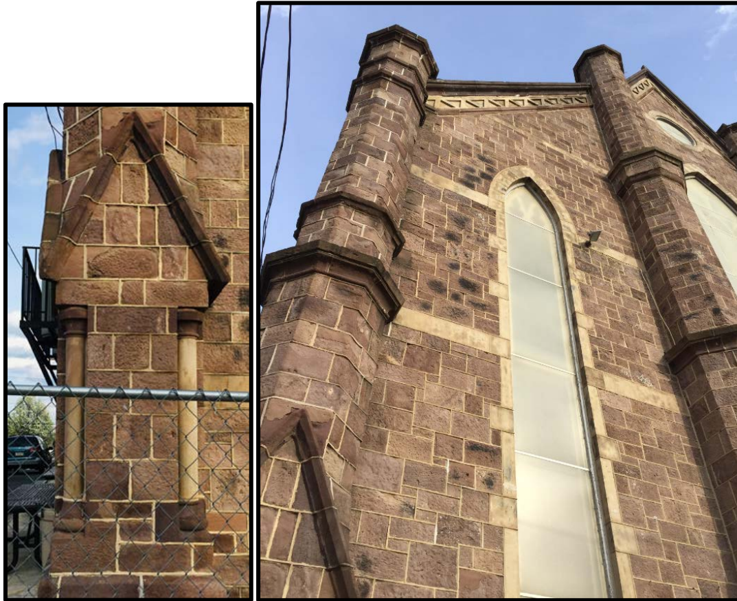
Figure 20. Left: A detail shot of the buttress at the base of the octagonal turret at the northwest corner of the building, showing its gable-front supported by colonettes. Figure 21. Right: The primary (west) elevation of the subject property, showing the northern most bay with a pointed arch window, a window hood, an octagonal tower and pilaster, and the Gothic-inspired cornice. Source: Oscar Beisert, 2019.
