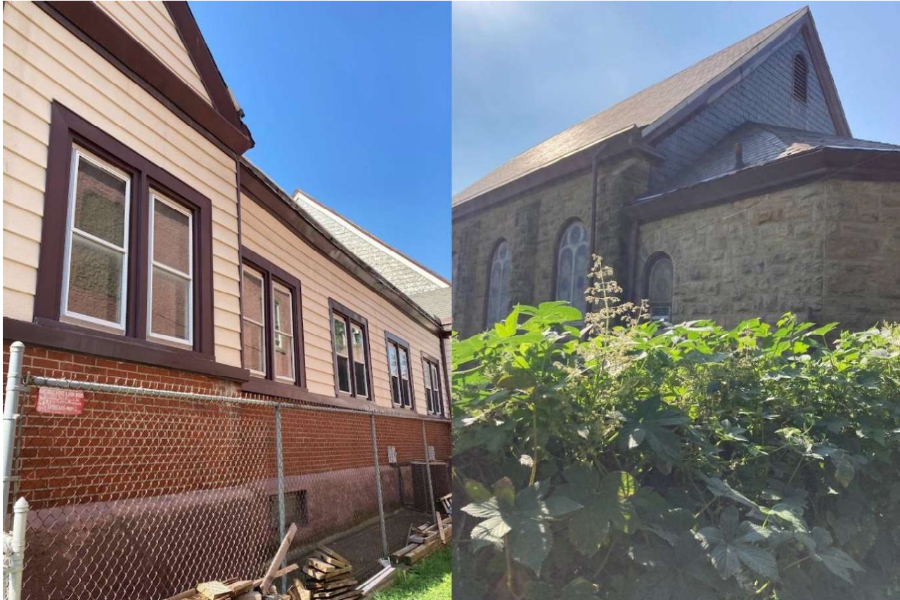
Figure 2: Left, Northeast Side from the Southeast corner. Right, Northeast side from the Northeast corner. Photos taken by Amarynth Ruch
