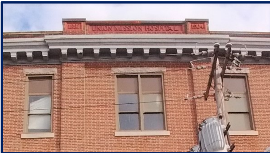
Figure 10: Detail of the cornice and parapet. The projecting cornice presents simplified classical molding over modillions.
