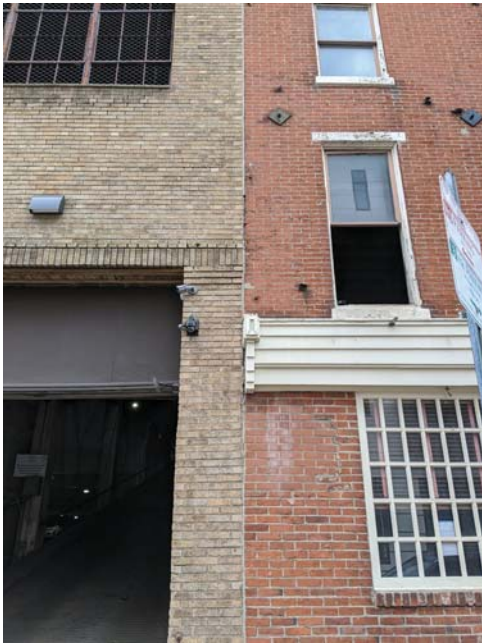
DIFFERING BRICKS & MORTAR JOINTS, REPLACEMENT CORNICE
