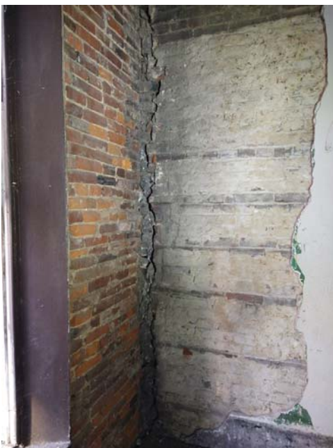
BRICK COLD CONNECTION AT FRONT FACADE
