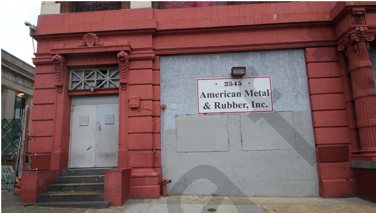
Photograph 2 – West elevation, Entrance detail, view east. Note the terra cotta detailing by the Conkling Armstrong Terra Cotta Company. The southern (right) bay was originally a window opening with a terra cotta sill. It was lowered in the mid- to late 20 th century for reasons unknown.
