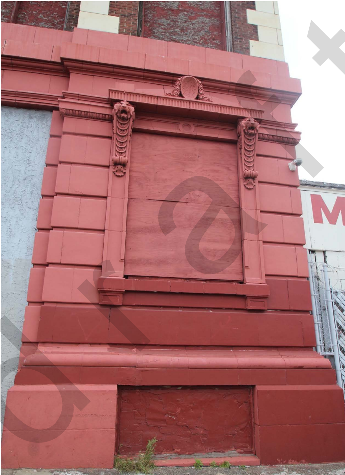
Photograph 4 – West elevation, Storefront detail, view east. Note the terra cotta detailing by the Conkling Armstrong Terra Cotta Company. The bay original contained a window.
