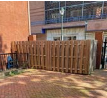
EXISTING 20TH C BRICK WALL, WOOD FENCE AND HVAC UNITS TO BE REMOVED
