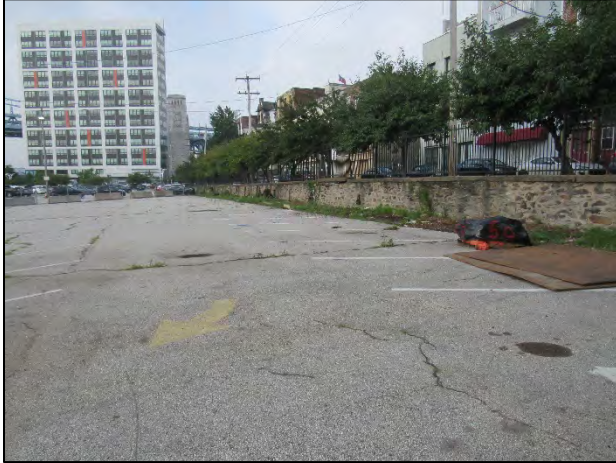
Photo 2.1. A view of the project area looking southwest toward the stone retaining wall along the edge of Water Street.
