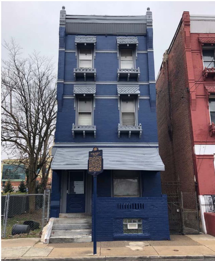
Figure 3: East-facing front façade along N. 23 rd Street, March 2021. Philadelphia Historical Commission staff.
