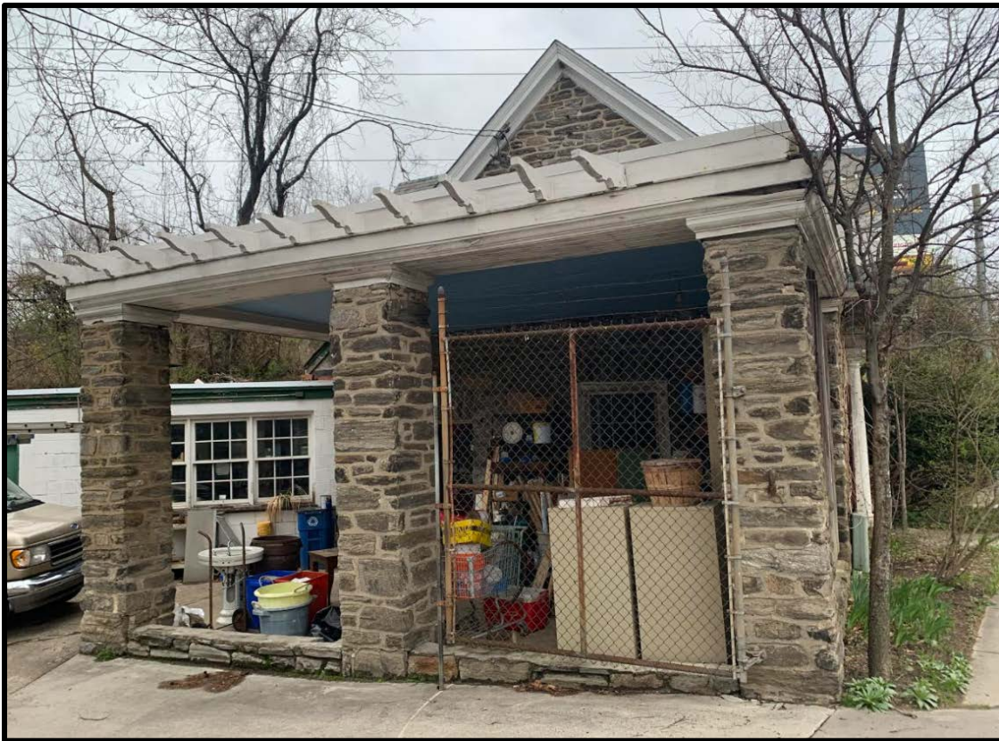
Figure 6. The south elevation, showing the porch styled to appear as a pergola. Source: Oscar Beisert, 2020.
