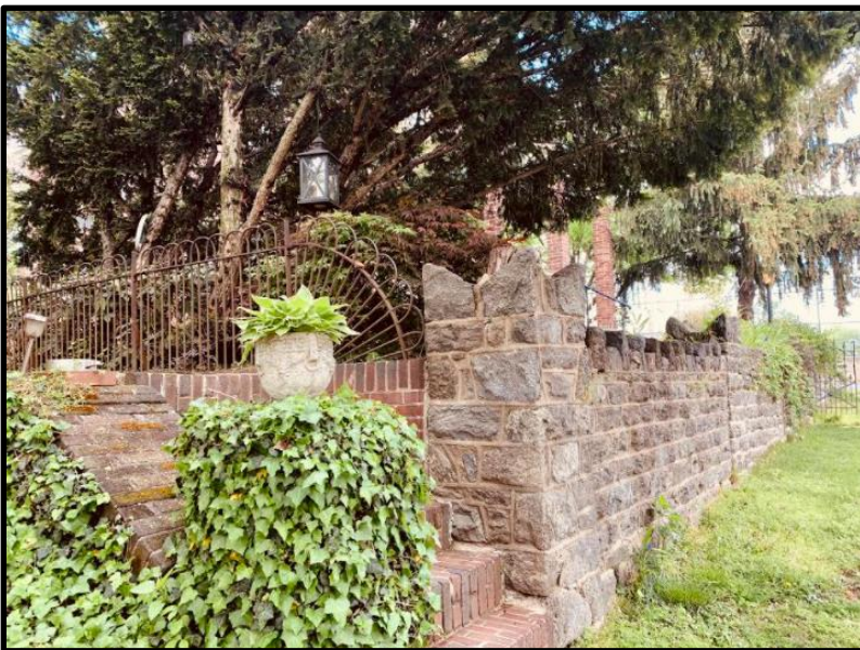
Figure 7. Top: Looking northeast, the stone retaining wall, yard, and front porch of the subject property. Figure 8. Bottom: Looking northeast at the iron fence and stone retaining wall at the south corner of the subject property. Source: Oscar Beisert, 2021.
