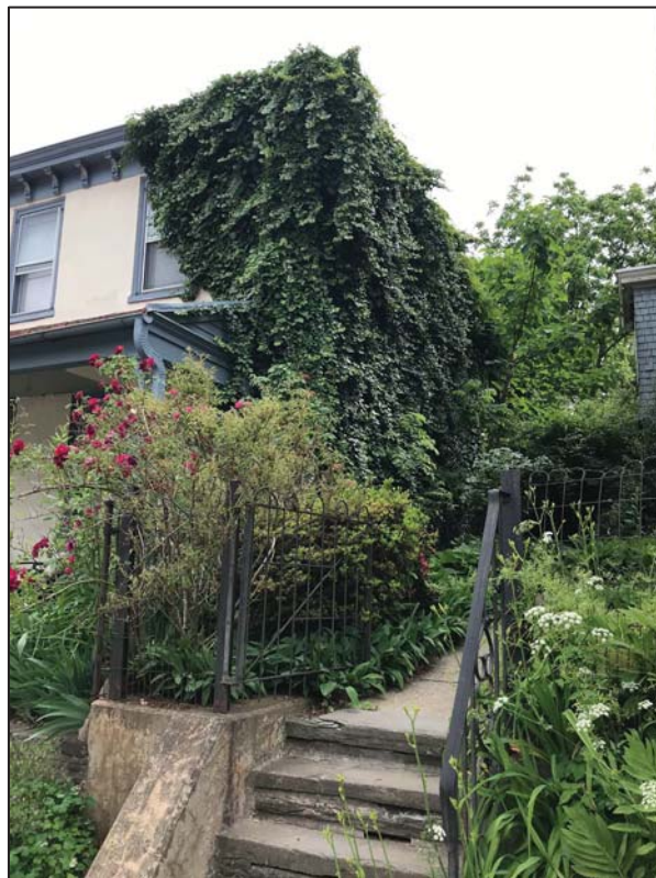
Fig. 10. The north elevation obscured by ivy and showing the front steps of the adjacent property.
