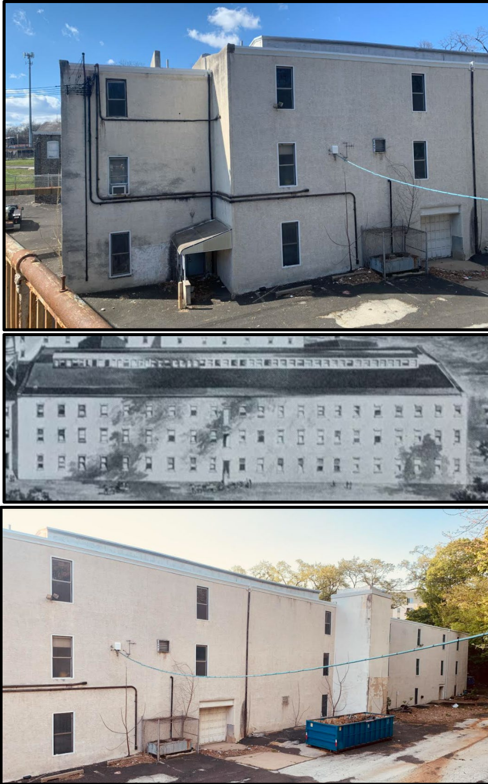
Figure 11. Top: The southeast elevations of Buildings 6 and 1. Source: Oscar Beisert, 2020. Figure 12. Middle: The southeast elevation of Building 1. Source: The Germantown Historical Society. Figure 13. Bottom: The southeast elevation of Building 1. Source: Oscar Beisert, 2020.
