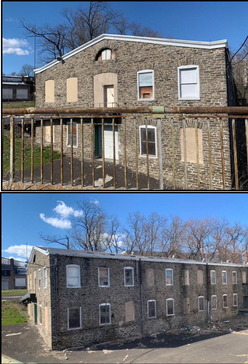
Figure 22. Top: The primary (south) elevation of Building 3. Figure 23. Bottom: The side (east) elevation of Building 3. Source: Oscar Beisert, 2020.
