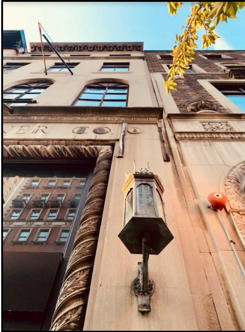
Figure 5. Details at the eastern extreme of the primary (south) elevation of the J.E.Limeburner Store. Source: Oscar Beisert, 2020.
