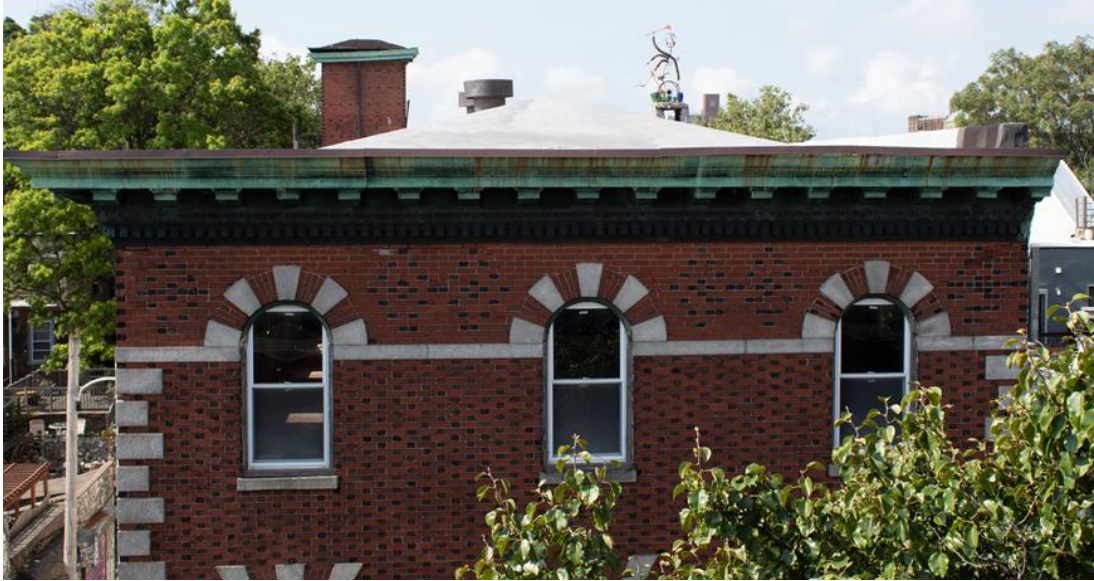
Figure 5 Detail, north elevation, third floor windows, 1016-18 South Street. Note use of modern double-hung windows. (Source: Author, 2020)
