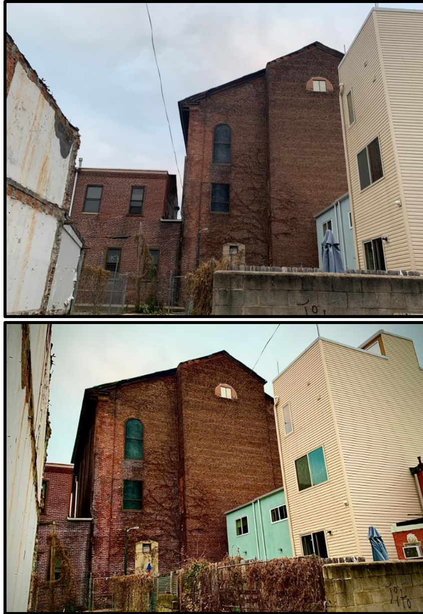
Figure 14. Top: The rear (south) elevation of the Main Block and the Chapel from Letterly Street. Figure 15. Bottom: Looking northeast towards the rear (south) elevation of the Main Block from Letterly Street. Source: Oscar Beisert, 2019.
