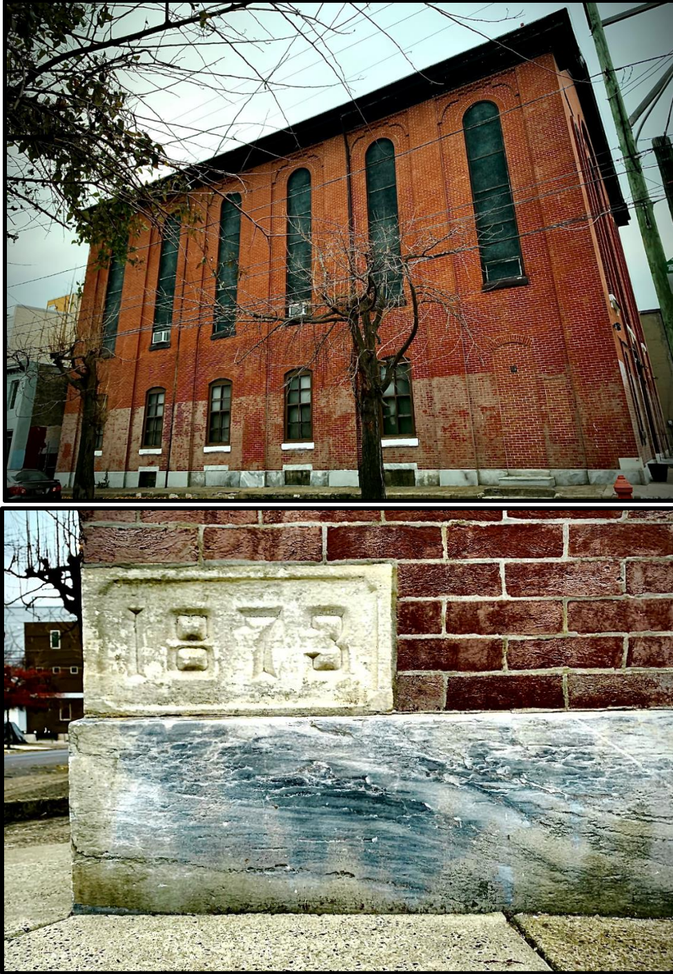
Figure 9. The side (east) elevation. Figure 10. The corner stone dated "1873." Source: Oscar Beisert, 2019.
