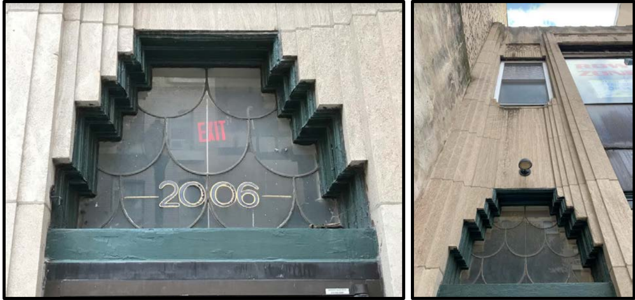
Figure 4. Left: The transom set defined by a ziggurat motif. Source: Tim Kerner, 2020. Figure 5. Right: The transom's ziggurat motif and its continuation into the second floor of the primary (north) elevation. Source: Oscar Beisert, 2020.
