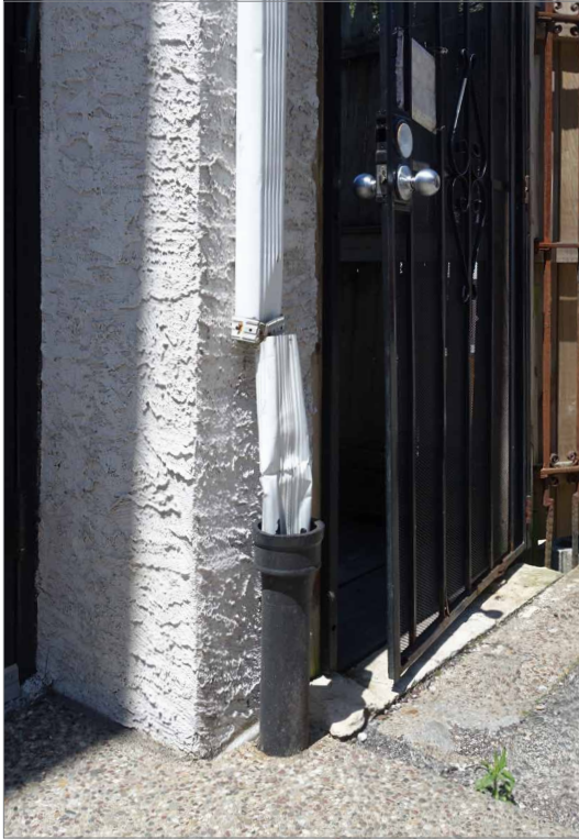
Downspouts should be maintained to direct storm water away from a building.
