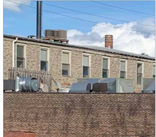
Elevating mechanical equipment at least 18” above the BFE or placing it on a rooftop can help protect it from damage from floodwater. Every effort should be made to minimize equipment visibility.
