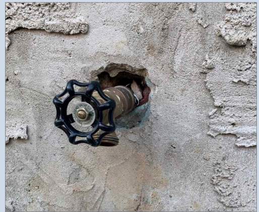
Sealing opening around penetrations such as hose bibs is recommended to reduce floodwater seepage.
