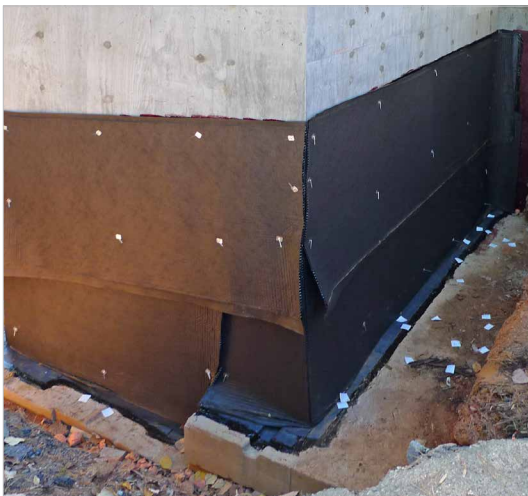
Concrete buildings are generally good candidates for dry floodproofing because of their ability to withstand loads and their smooth surface facilitates the application of sealers.
