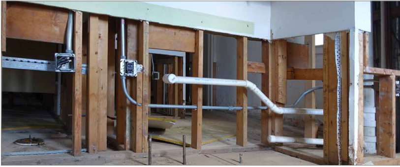
Interior drywall was removed and electrical outlets and plumbing connections were raised following a flood.
