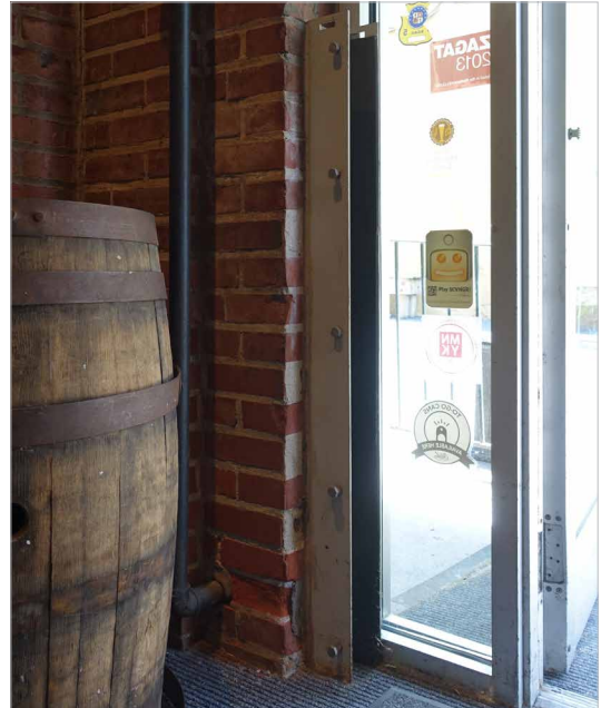
After persistent flooding, the building owner installed a flood barrier at the inside of the entrance door. When a flood occurs, panels are inserted into the channel and the glass doors are opened to prevent the water pressure from shattering them.
