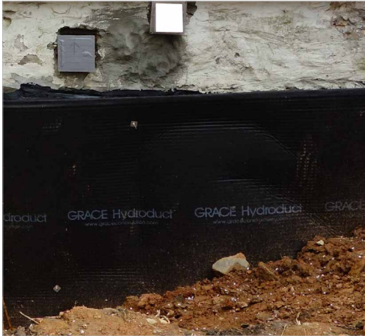
The structural integrity of masonry walls should be verified prior proceeding with dry floodproofing. All sealers should be concealed by soil or historically appropriate material based upon location.
