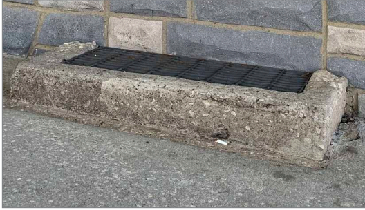
A curb around a basement window openings can serve as a barrier to floodwater.
