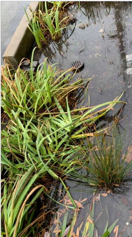
Rain gardens on Venice Island collect stormwater from the parking lot and then slowly allow it to be absorbed into an underground storage tank.
