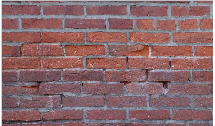
Delaminated bricks and open joints in a brick wall can provide a pathway for floodwater into the building. Regular maintenance can preserve the wall and improve its long-term performance.
