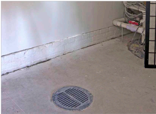
Accumulated flood water is evacuated through floor grates and a sump pump, whose piping is partially concealed by the screen.
