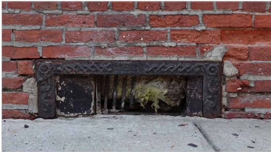
For dry floodproofing, basement level windows located at or near the ground will need to be infilled to create a water tight barrier. The repair and repointing of the surrounding brick will also improve the building's flood resilience.
