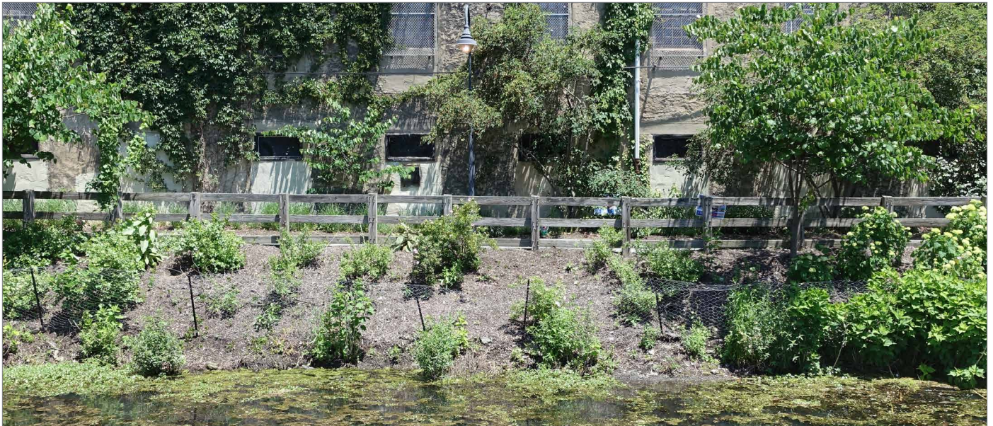
Partially sealing the lower portion of the ground floor windows may serve to slow floodwater infiltration from the river and canal.
