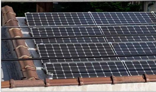
Solar panels can provide an alternative source of electricity after a flood to power sump pumps and fans.
