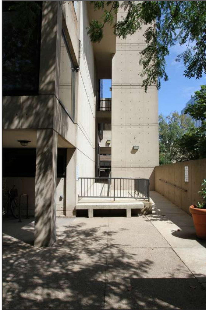
Figure 32: Partial view of the east facade of the International House, showing the enclosed exit stair that is connected to the main structure by a narrow bridge at each level. (Source: Allee Davis, August 2019)
