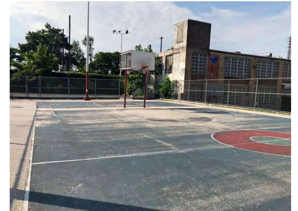
Basketball courts are popular and could use new surface paint
