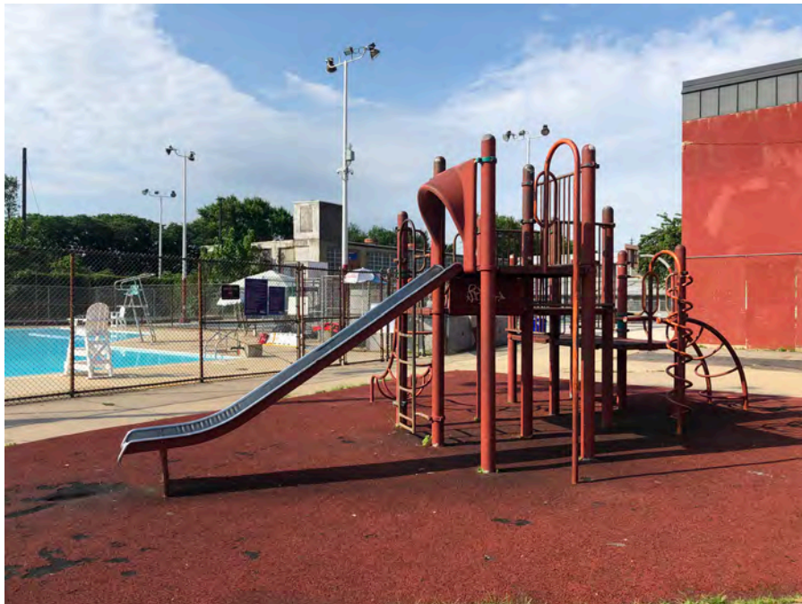
Play equipment is old and needs to be replaced
