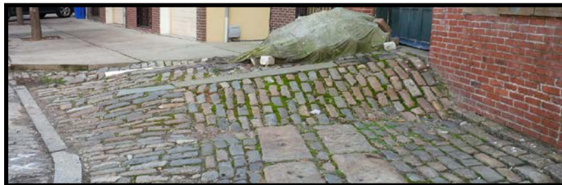
Figure 7: The pavement in front of the building's eastern block. Source: Michelle Shuman, 2018.
