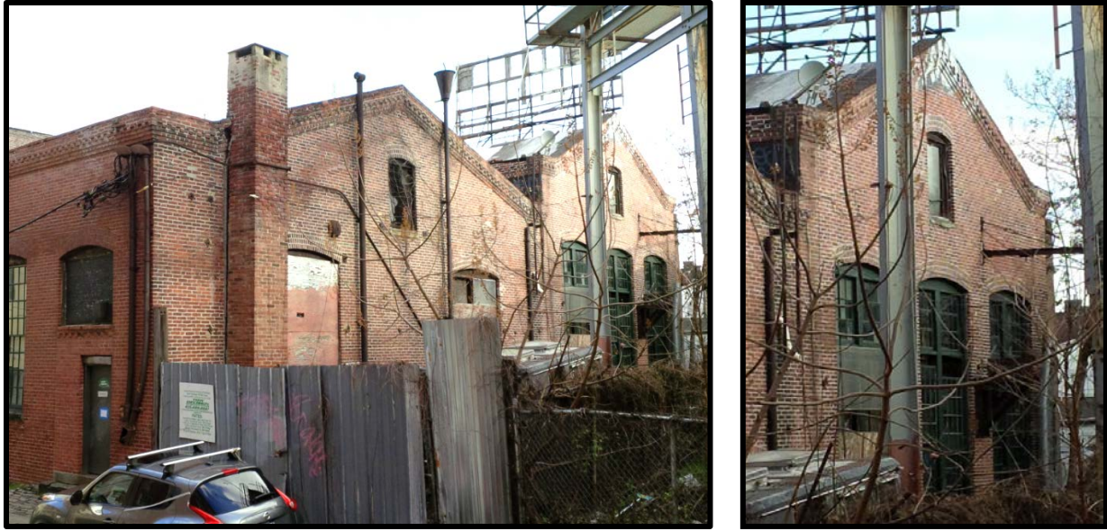
Figure 13: Left: View from Sarah Street of the west and rear (south) elevations of Building 10. Right: Detailed view of the eastern block's rear, featuring original and/or early windows and doors. Source: Michelle Shuman, 2018.
