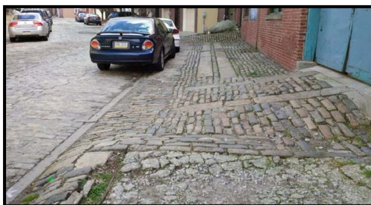
Figure 9: The pavement in front of the north elevation of Building 10. Source: Michelle Shuman, 2018.
