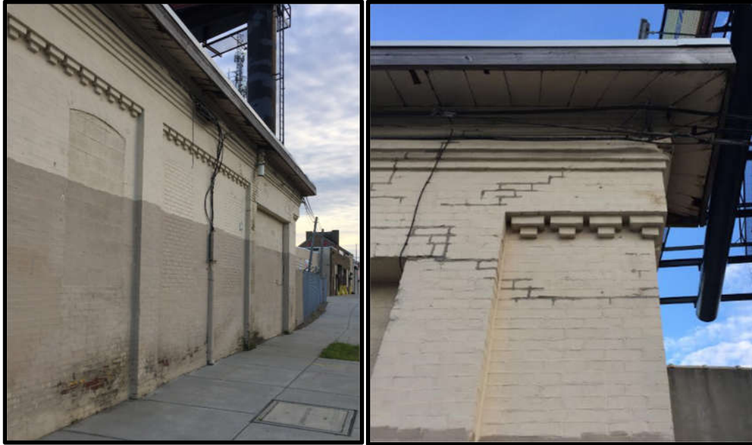
Figure 4. Top left: The primary (northwest) elevation. Figure 5. Top right: Cornice details of the primary (northwest) elevation.
