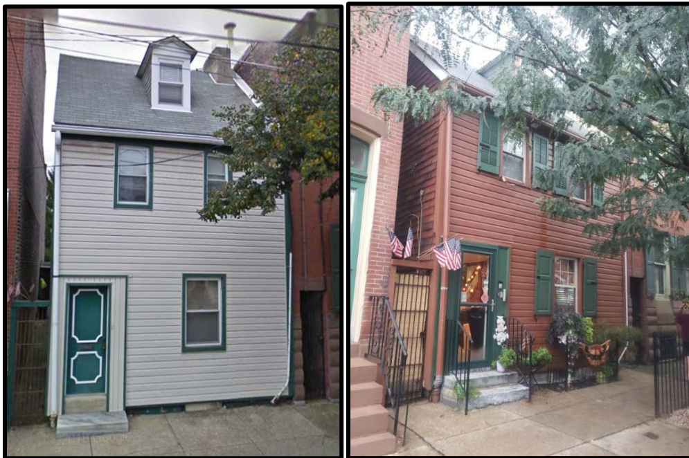
Figures 20 and 21. The above photographs show 1112 Marlborough Street before (left) and after restoration. The frame dwelling is a great example of what can be done to restore a period appearance to a wooden house with some relaxed standards. While the windows and siding appear to be of faux materials, the overall appearance of the house after renovation (right) has a historic quality. The 2009 Google Street View photograph (left) shows a much more mundane view of 1112 Marlborough Street. By 2013, Google Street View shows that house had been renovated to its present appearance (photograph on right taken in 2019). This building also appears to be of a similar wooden house form and scale as the subject property.
