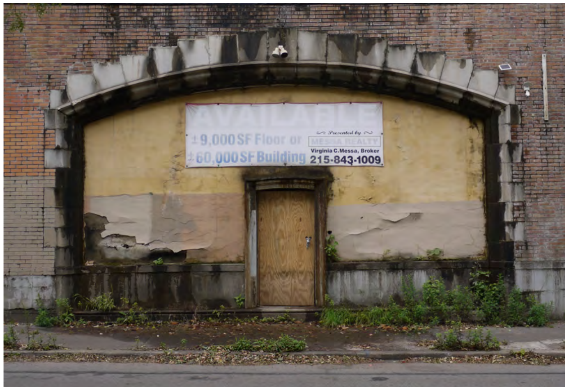
Figure 9. Detail view of the entrance on the southeast façade of the Germantown Fireproof Storage Company building.
