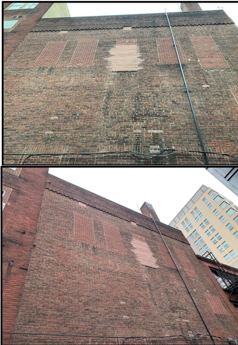
Figure 8. Top: The rear (north) elevation of the subject property. Figure 9. Bottom: The rear (north) elevation of the subject property. Source: Oscar Beisert, 2019.
