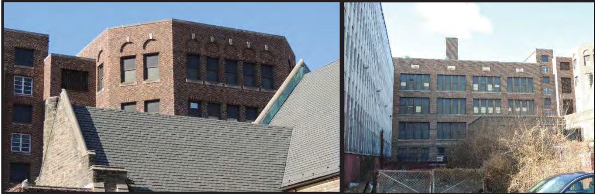
Figure 34. Above: Looking west at the site of Germantown High School. Source: Atlas, City of Philadelphia, 2018. Figure 35. Below: the southeast elevation of the 1913–14 Building, specifically the central portion. Right: The rear (southeast) elevation of the 1913–14 Building, showing the southwest wing. Source: Nicholas Covolus, 2018.
