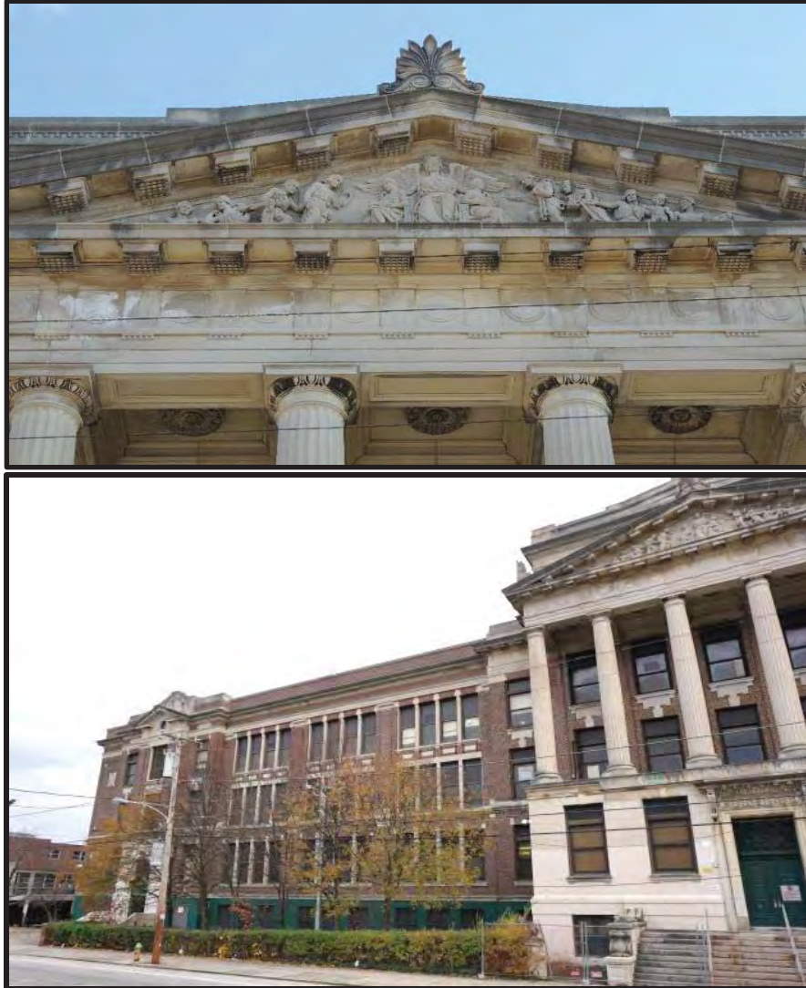
Figure 22. Top: The pediment within the primary (northwest) elevation. Source: Nicholas Covolus, 2018. Figure 23. Bottom: The northeastern portion of the primary (northwest) elevation. Source: Oscar Beisert, 2018.
