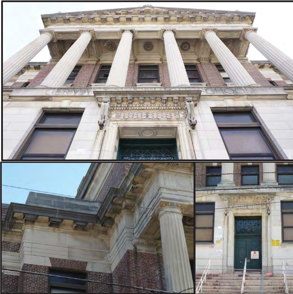
Figure 19. Top: Looking upwards towards the ceiling of the portico on the primary (northwest) elevation. Source: Oscar Beisert, 2018. Figure 20. Bottom left: Cornice detail on the 1913–14 Building. Figure 21. Bottom right: the architectural details of the central entrance within the primary (northwest) elevation. Source: Nicholas Covolus, 2018.
