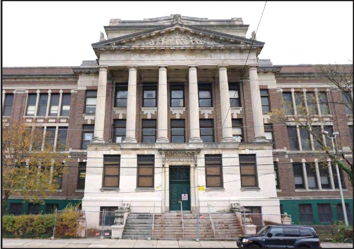
Figure 18. The portico and central pavilion of the primary (northwest) elevation. Source: Nicholas Covolus, 2018.
