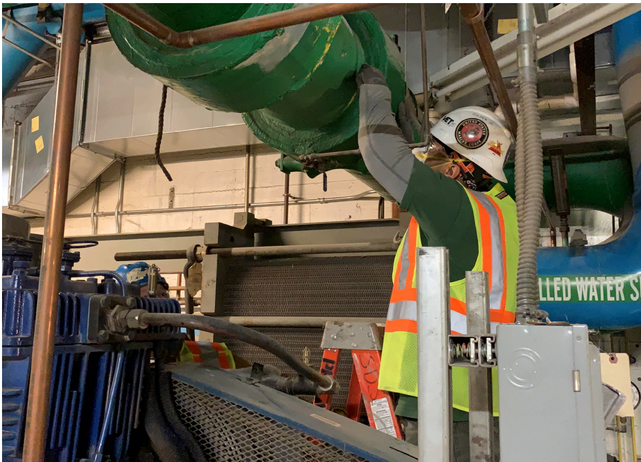
Workers installing a new energy efficient chiller at the Philadelphia Museum of Art.
