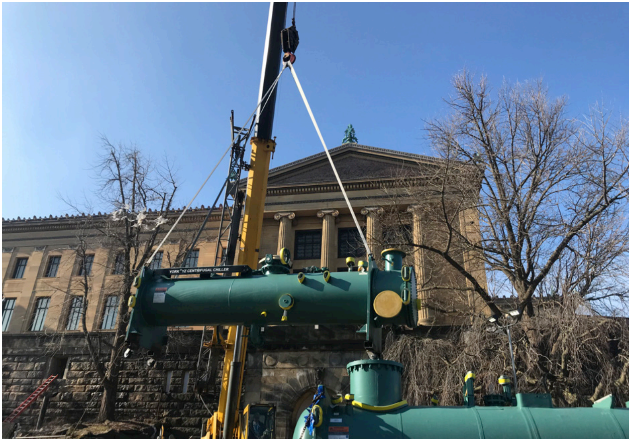
Workers outside the Philadelphia Museum of Art lift a new high efficiency chiller off the delivery truck.
