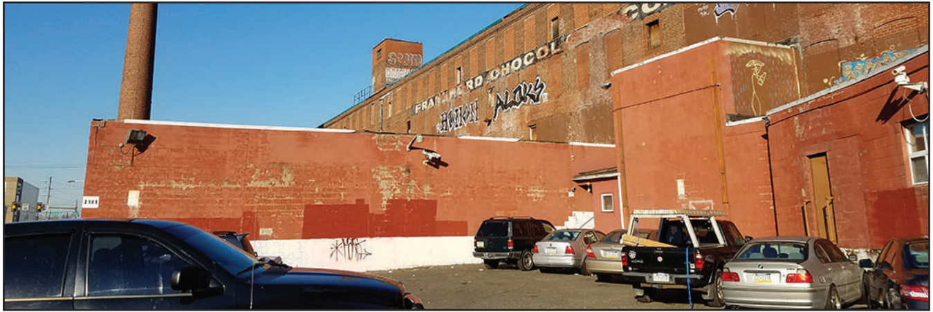
Figure 17: East elevation of 1967 Addition A with a portion of 1967 Addition B | Photo: Dennis Carlisle
