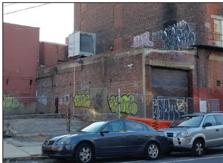
Figure 10: The only segment of 1912 Addition B visible from street level. | Photo: Dennis Carlisle
