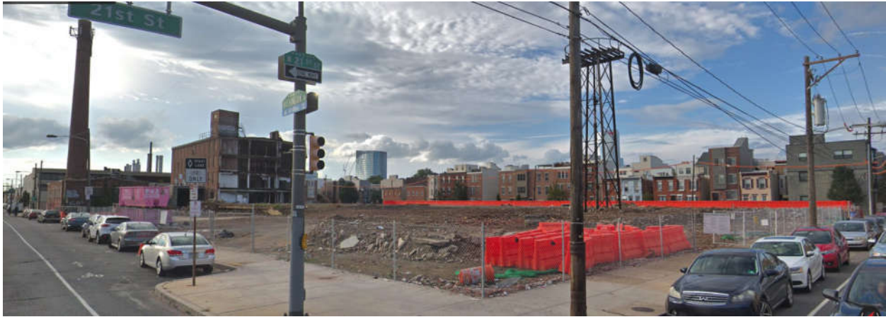
Figure 5. Looking to the northwest at the site from the corner of 21 st Street and Washington Avenue, September 2018. Note that the smokestack was demolished after this photograph was taken.
