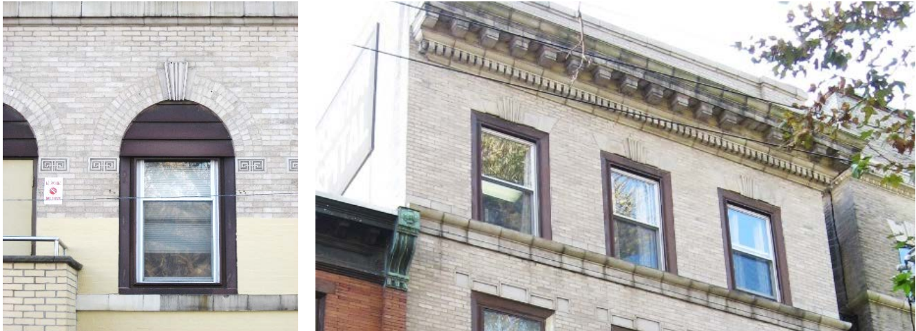
Figure 16: Left, first-floor window opening detail. Right, details of the cornice and parapet and ornament above 3 rd and 4 th -floor windows.
