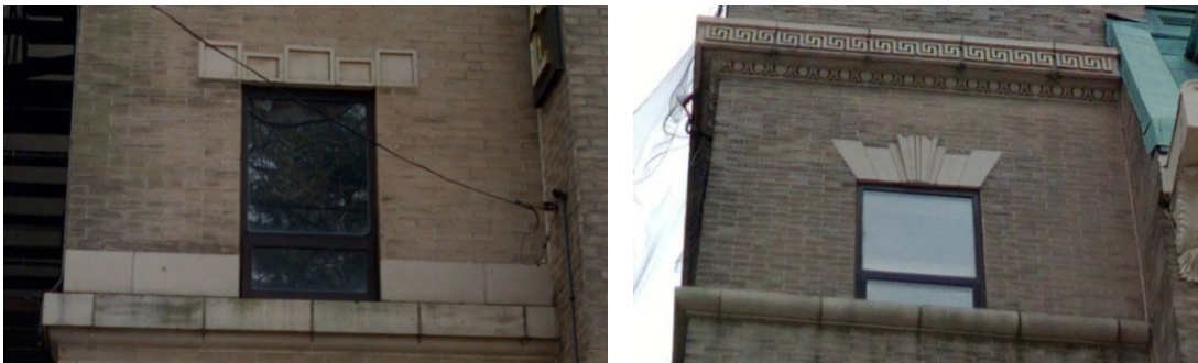
Figure 14: Details of the second and fourth-floor window openings, beltcourses, and terra cotta detailing.
