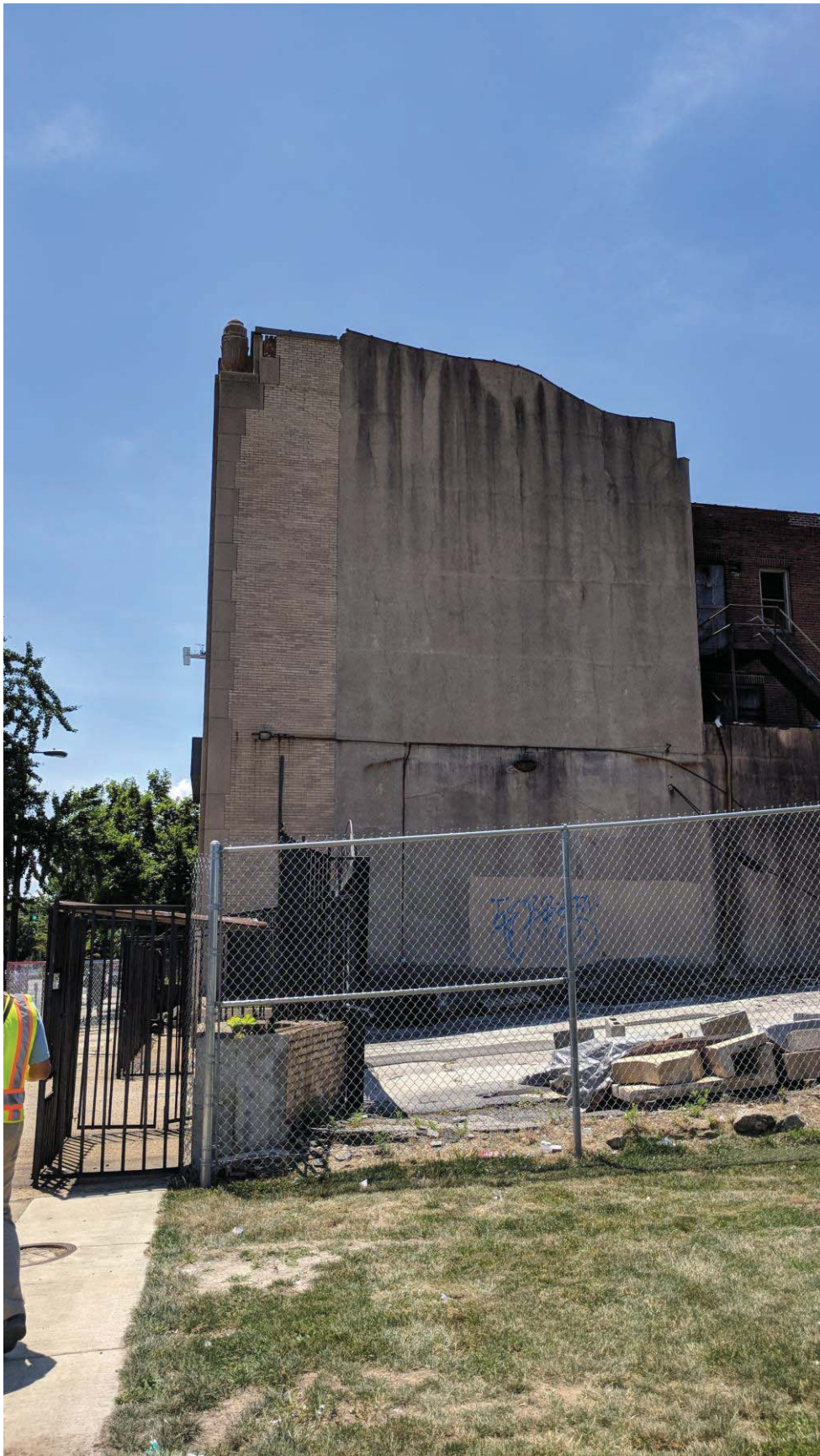
Photo No. 6. Loose masonry and decorative pieces at roof level
