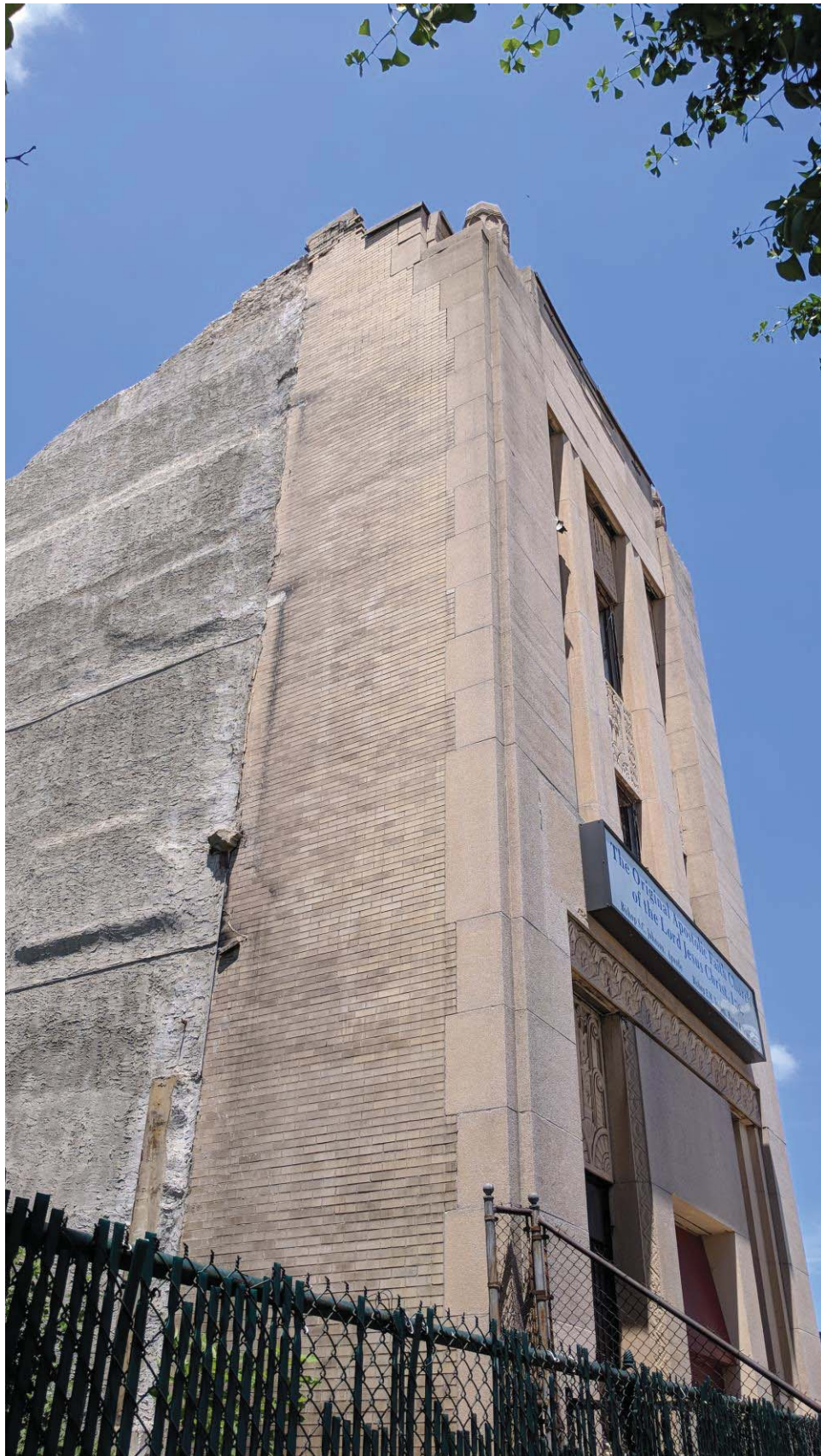
Photo No. 8. Loose masonry and decorative pieces at roof level
