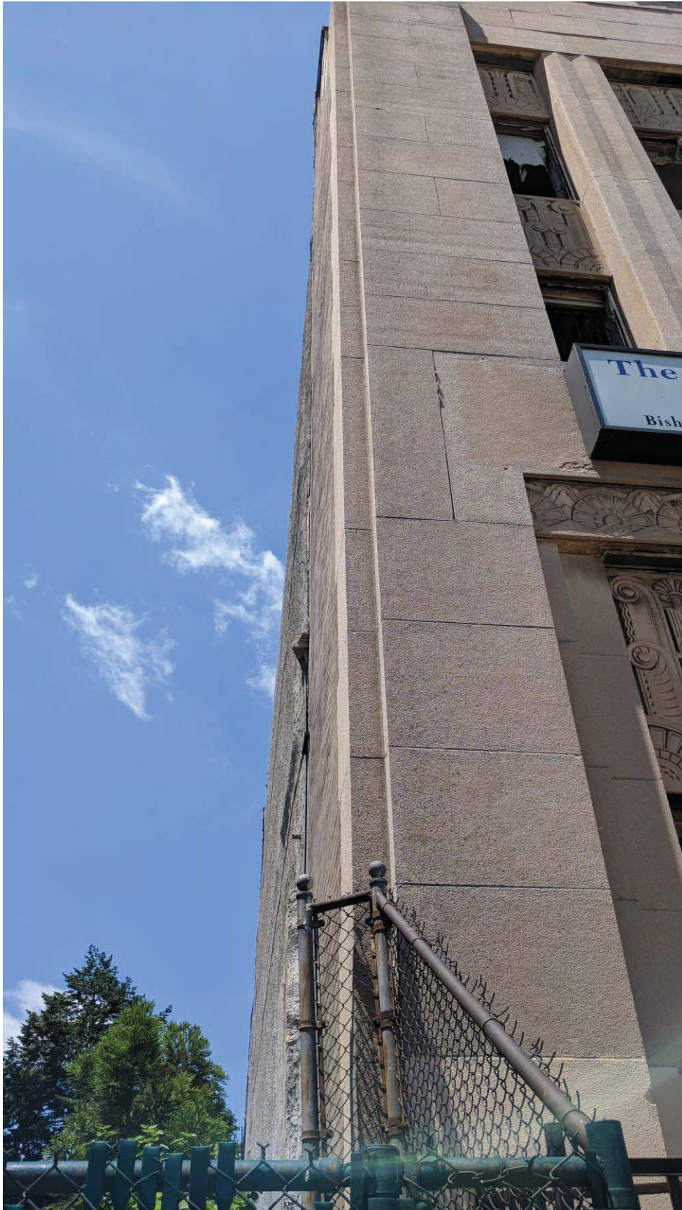
Photo No. 3. Some bulging noted at south wall
