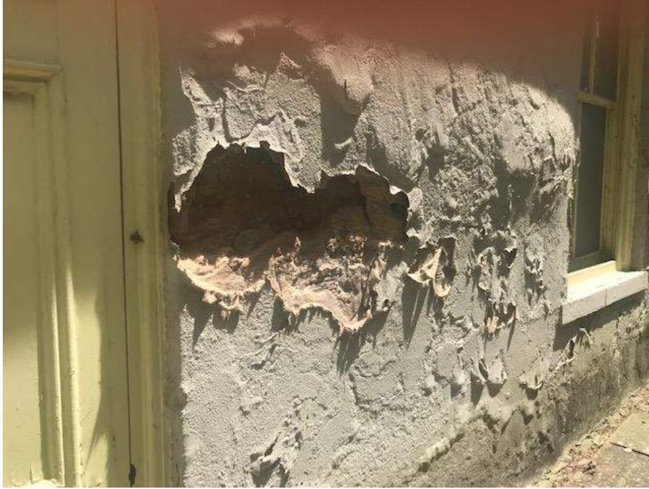
Shed exterior, stucco over rubble stone; extensive water damage stucco turning to dust behind waterproof coating
