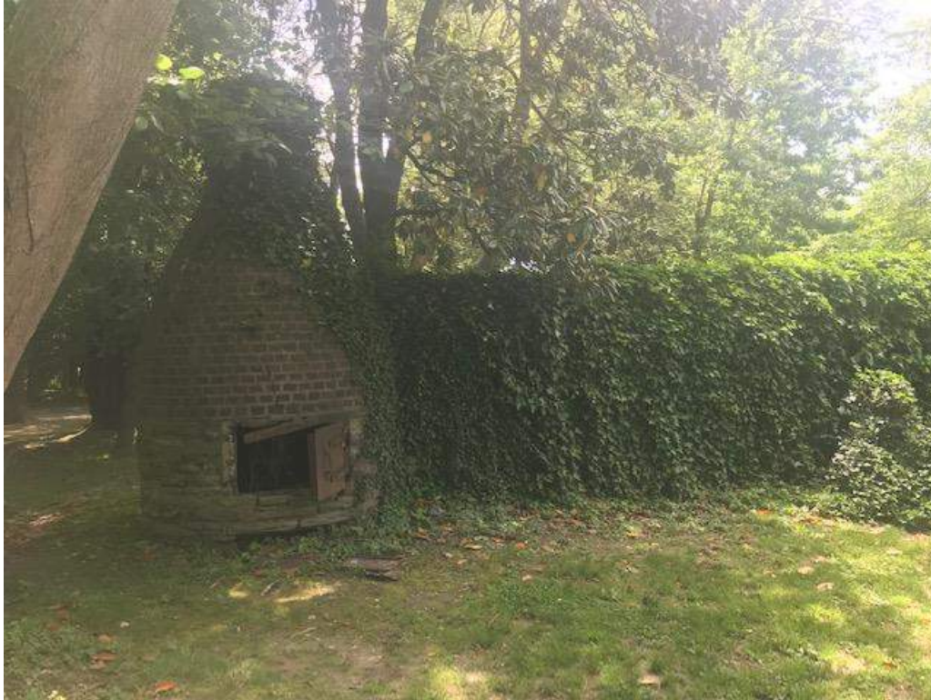
Incinerator and wall, extensive damage to incinerator and masonry above
