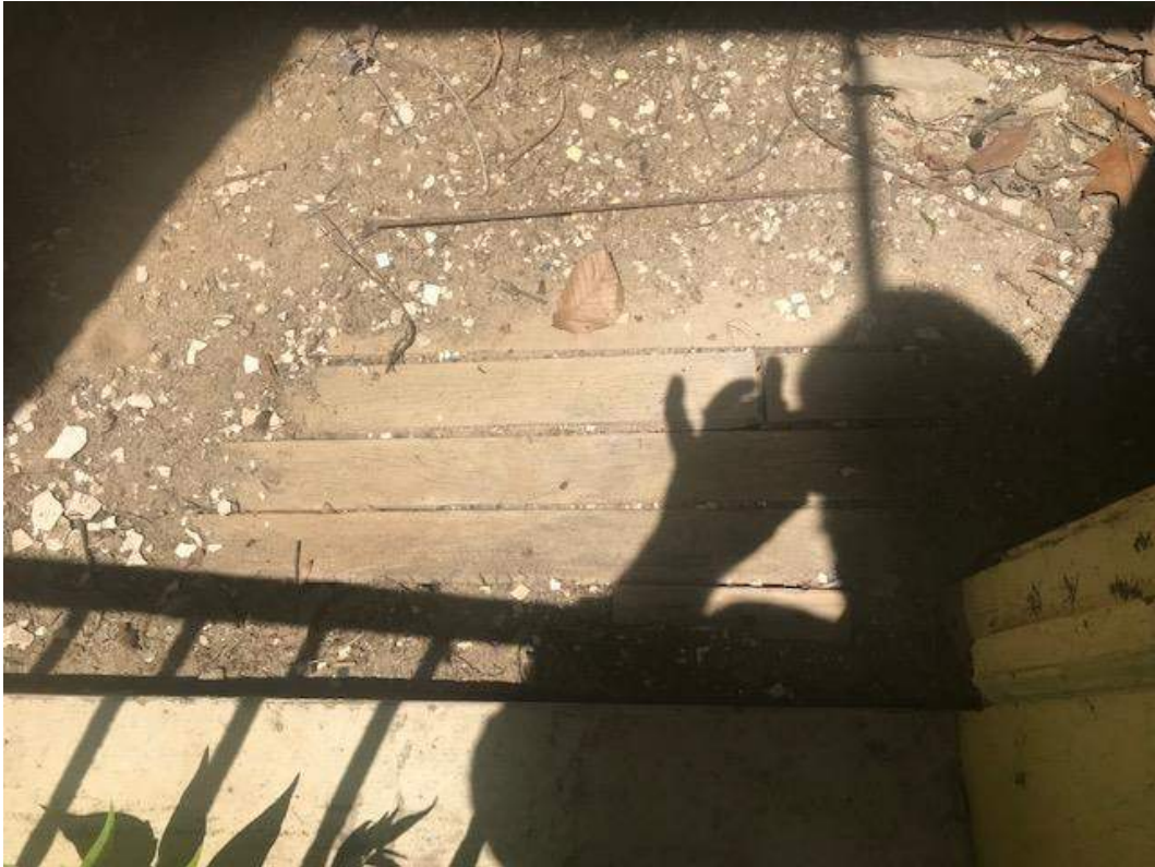
Shed – rotted floor, door frame termite damage lower right
