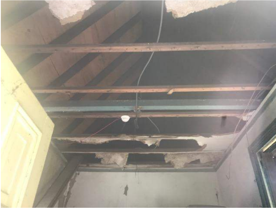
Shed interior, rebuilt interior roof; ceiling collapsed
