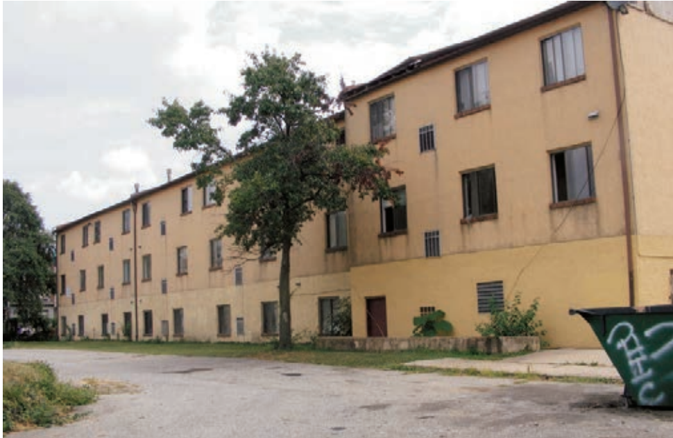
Left: Damaged roof and gutters contributes to water problems both inside and out. Signs of mold and mildew are evident along the exterior of the buildings.
