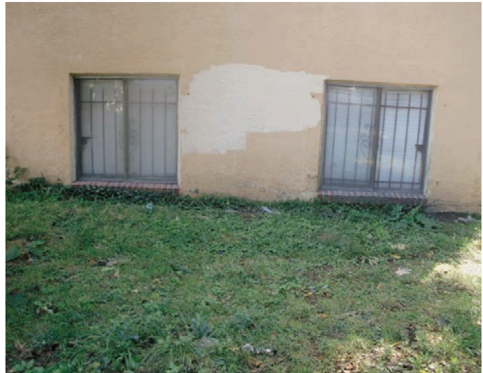
Right: Windows at ground level create damp conditions inside units creating conditions which promote the growth of mold and mildew. The at-grade windows also cause concerns for privacy and security
