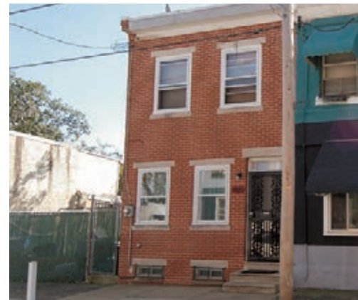
Left: Rehabilitation of existing housing stock removes blighted properties from the neighborhood and can provide an affordable option to residents
