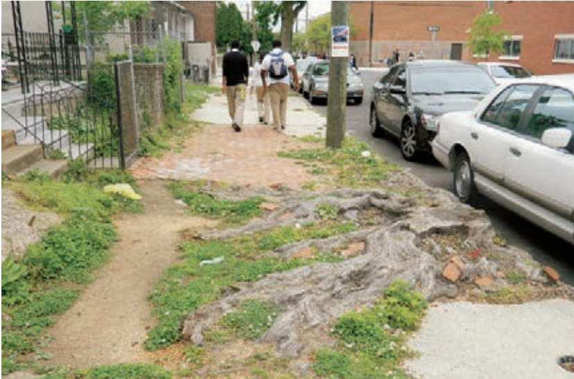
Example of sidewalk conditions in various sections of the West End
