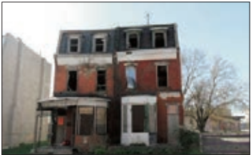
Vacant residential structures
