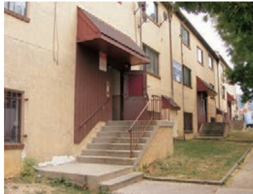
Far left: Damaged gutters dump water at the foundation of the buildings, undermining the structural stability
