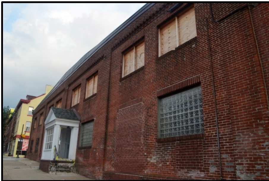
The Chestnut Street elevation of Building No. 3 with the vestibule addition. Source: Oscar Beisert, 2018.
