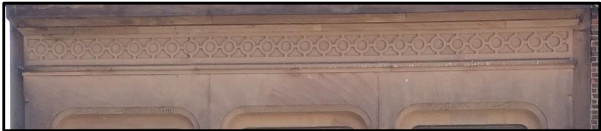
Figure 8: The cornice of the primary (north) elevation of 726 Chestnut Street. Source: Oscar Beisert, 2018.
