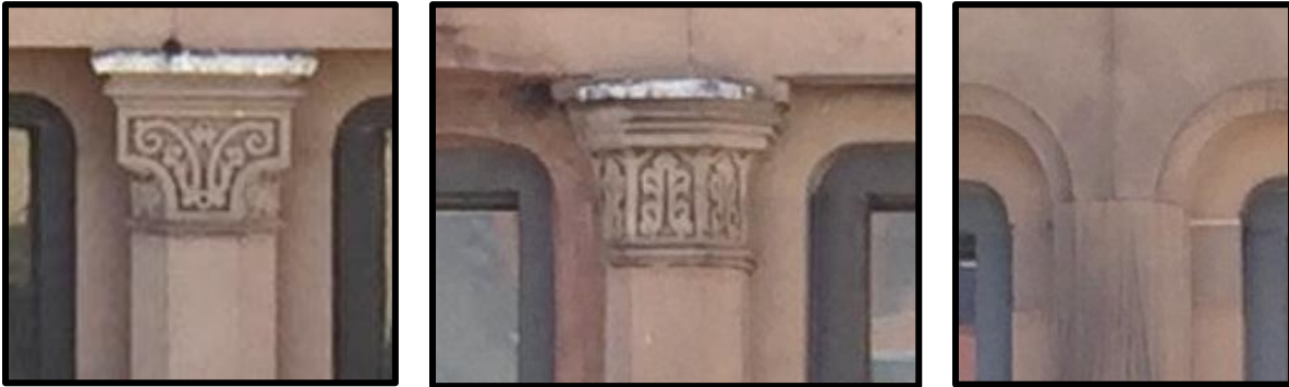
Figure 7: Capitals on each floor of the primary (north) elevation of the building, from second to fourth, left to right. Source: Oscar Beisert, 2018.
