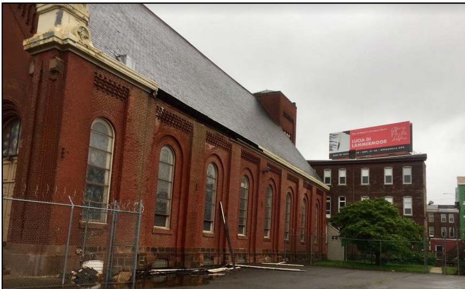
Figure 7: West elevation of the Church and north elevation of the Rectory. Source: Oscar Beisert, 2018.
