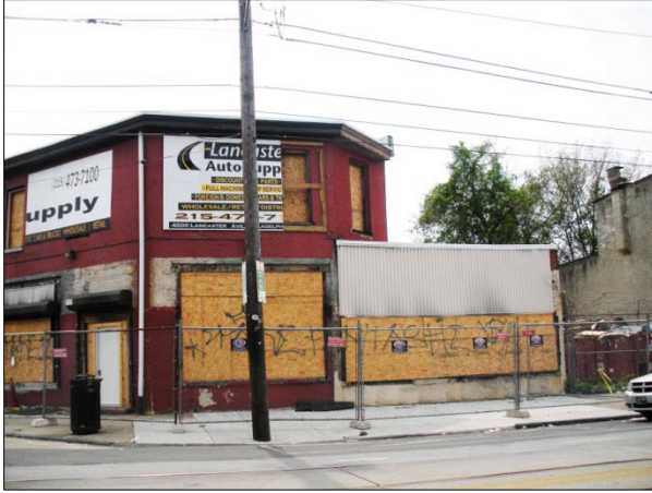
Vacant buildings and a vacant lot at the corner of Lancaster Ave and 45 th St. Again, plywood and a fence are all that prevent entry in the vacant buildings and trash has accumulated in the vacant lot.
