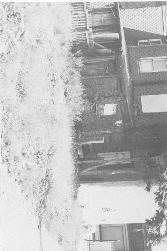
A dilapidated structure 4700 block of Bermuda Street
