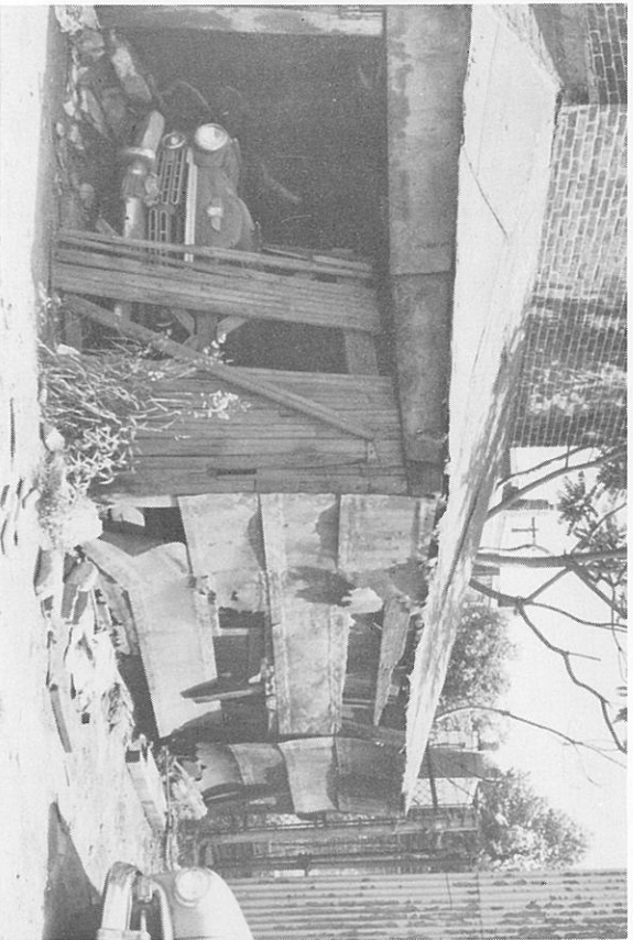
A dilapidated structure 2300 block of Pratt Street
