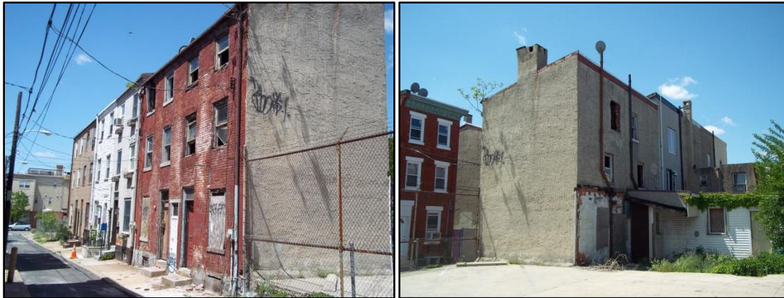
These houses on the 200 block of W. Stiles Street have broken and boarded windows and doors, holes in the back wall, and graffiti. Loose bricks have fallen off of the front wall of one property and lie on the sidewalk next to the stoop.
