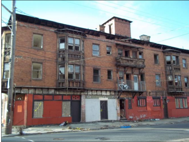
This vacant building is the only thing standing on the block bounded by 21 st Street, Ridge Avenue and Oxford Street. The open door and broken windows and trash show that someone has recently accessed the property. This is a public safety concern
