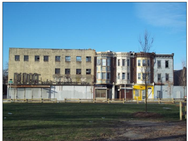
The vacant buildings in the background are in the 2000 block of Ridge Avenue. Only two buildings on the block are occupied. Notice the sky showing through the large building on the left.
