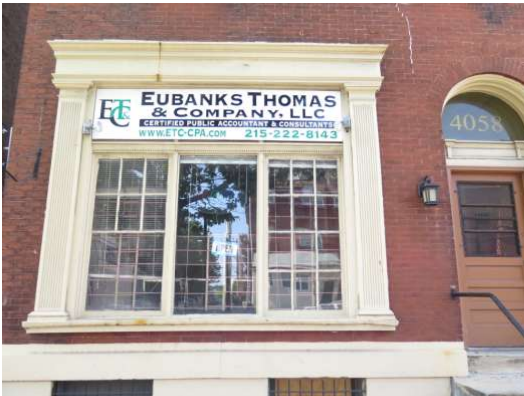
Figure 8. Casement window on the ground floor of 4058 Chestnut Street. Source: Kelly E. Wiles.
