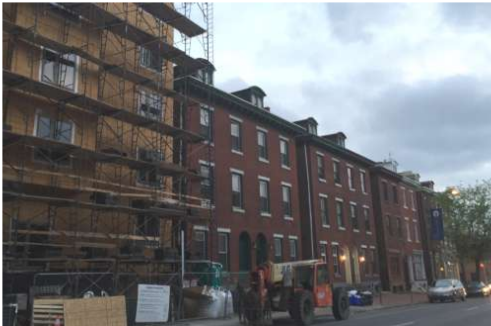
Figure 4. Looking southwest. The buildings in the foreground, 4046-48 Chestnut Street, were demolished in 2016. Source: Oscar Beisert.
