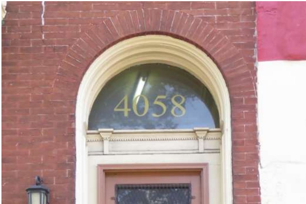
Figure 10. Door surround of the entrance at 4058 Chestnut Street. Source: Kelly E. Wiles.
