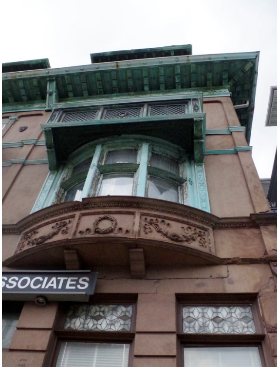
A view of the copper details at the façade of the property at 2305: an oriel window at the piano nobile, capped by a decorative balcony and a heavy, bracketed cornice below a mansard roof at the fourth floor. Photo: Author. Juliet
