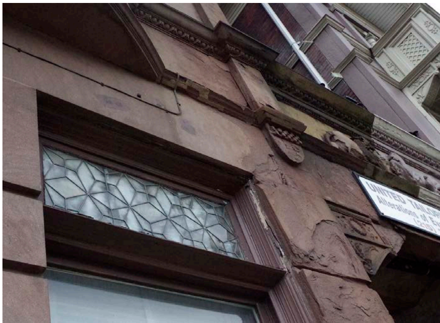
A close up of a transom window at 2305 with lead coming in a Moorish pattern and a view of the brownstone deterioration at the connecting archway. Photo: Author.
