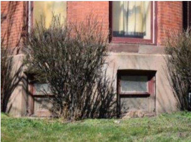
Figure 3: Portion of water table at base of east elevation and southeast corner of building that has been refaced with smooth cement.
