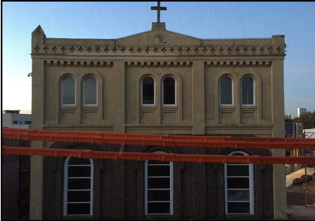
Looking south at the second and third floor façade of the primary elevation from the building opposite. Source: Oscar Beisert.
