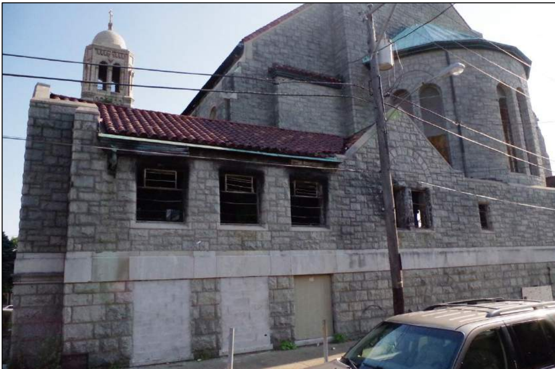
Fig. 9. North elevation of the church showing fire damage.
