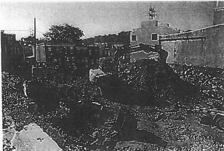
Among Philadelphia job sites where inspectors did not check on demolitions as they were in progress was 131 Shurs Lane in Manayunk, where a VFW hall and a parking lot were taken apart, inspectors said. CLEM MURRAY / Staff Photographer
