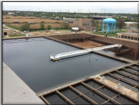
Figure 5: New Ferric Tanks and Chemical Feed system
