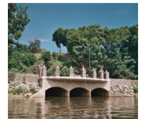
Dobson's Run Outfall (Source: PWD)
